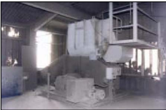
Inside the cement plant, the Dalamatic dust collector vents the elevator casing & cement discharge point.
